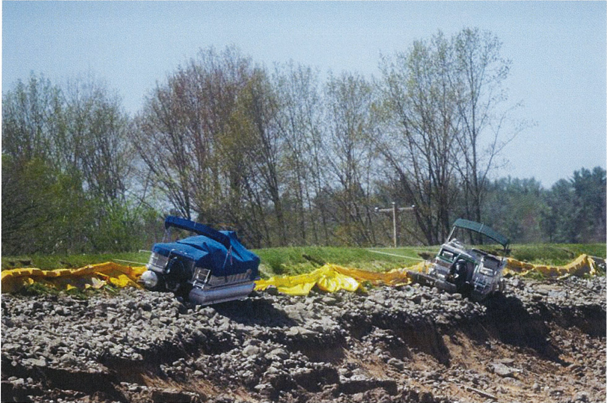
Two boats sit atop what remains of the Edenville Dam, washed up after severe flooding on Wednesday, May 20, 2020. 69
