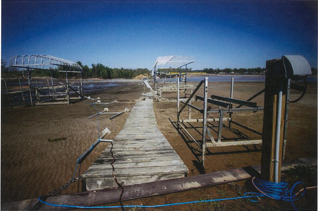
Washed out boating docks on Wixom Lake due to the failure of the Edenville Dam on Wednesday, May 20, 2020. 68
